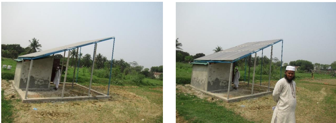
Fig 1. Solar pump installed at CA Park.
