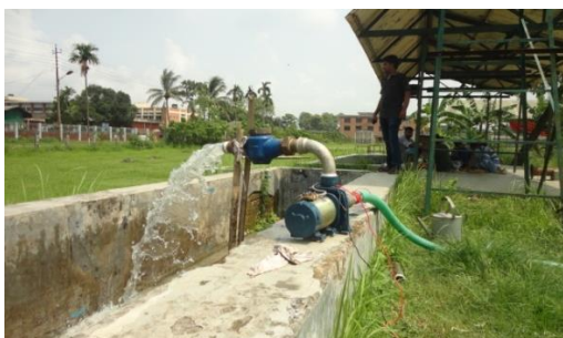
a. Large solar pump (910 W, 180 L/min)
