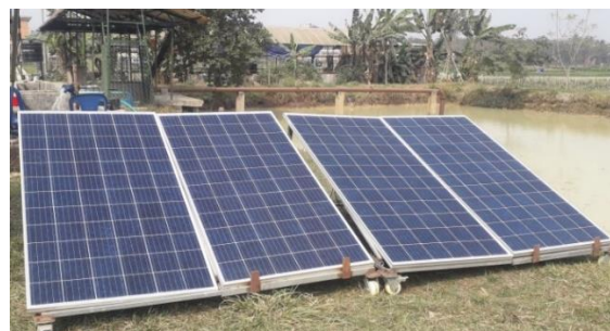
b. Solar panel (1300W @325W)
